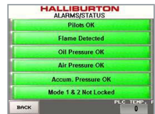
HMI Display screen for visual alarms
