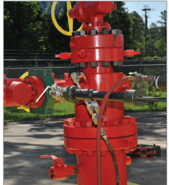
Engineered saddle for flange access to monitor annular pressure.
