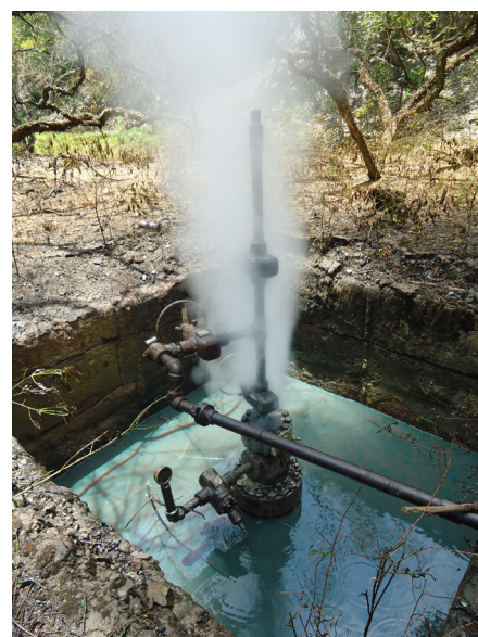
The remote well was leaking through the wellhead via the short string of a dual completion.
