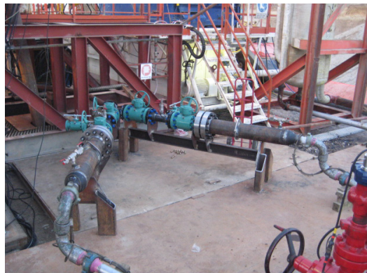
Rock catchers on the choke line
