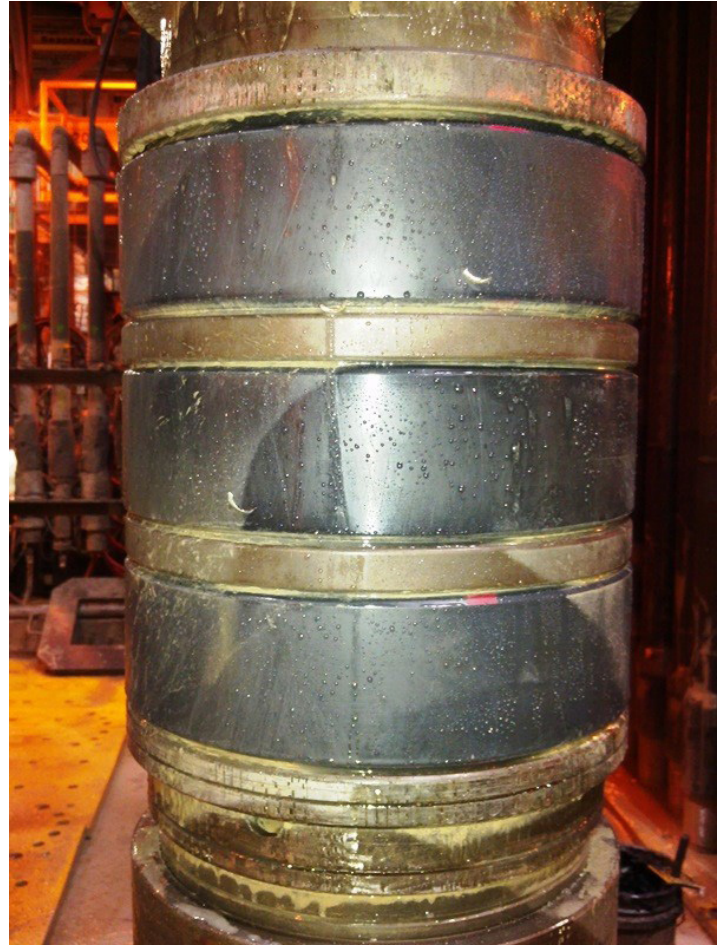
After being pulled out of hole, these packer elements are still in good condition.
