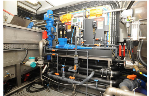
Pipe flocculator with chemical dosing system
