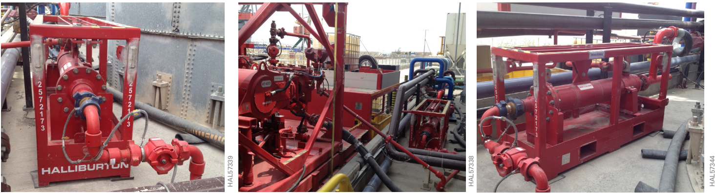
Skid-mounted, soundproofed Halliburton high-pressure shear unit installed at the LMP
