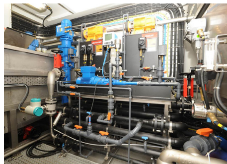
Pipe flocculator with chemical dosing system
