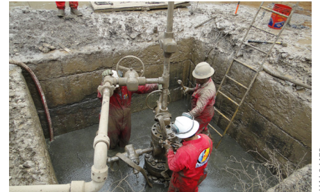
After regaining control of the well, the Boots & Coots team installed a new wellhead.
