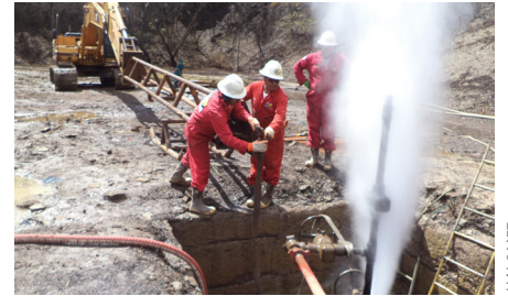
Prior to killing the leaking well, the Boots & Coots team had to first regain control of the well.
