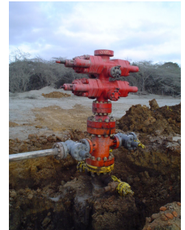
Boots & Coots installed a blowout preventer (BOP) stack on the well, and diverted gas flow to a burn pit.
