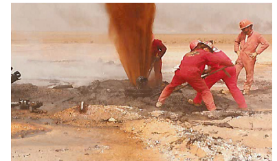
Figure 3. Well control experts with Boots & Coots work at close proximity to a wellhead, attempting to remove a flange. (Photo courtesy of R. Hatteberg)
